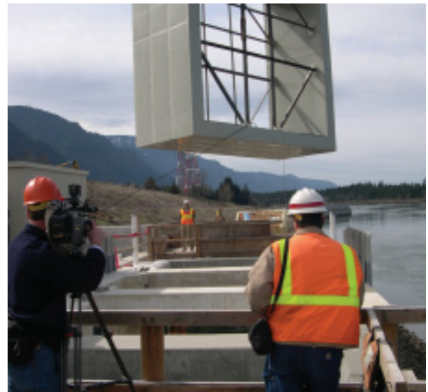
A portion of the world's largest radio frequency identification (RFID) antenna is lowered into place at the Bonneville Lock and Dam near Portland, Oregon
